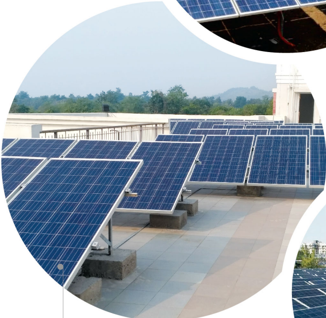
● 250 kW roof-top solar power plant & 425 kW of car port integrated solar power plant at Shrimad Rajchandra Trust - Dharampur, Gujarat
