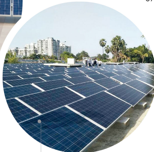
● Surat Municipal Corporation, Varied Waterworks Sites - 2 MW
